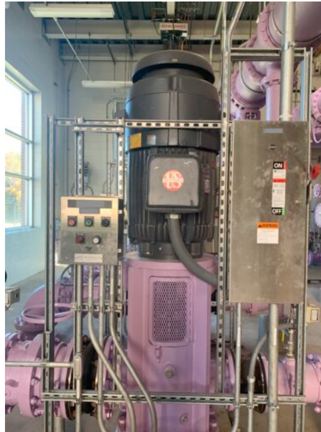
Figure 3: Totally enclosed, fan-cooled motor on variable frequency drive with winding thermal protection and safety disconnect. Courtesy: CDM Smith
