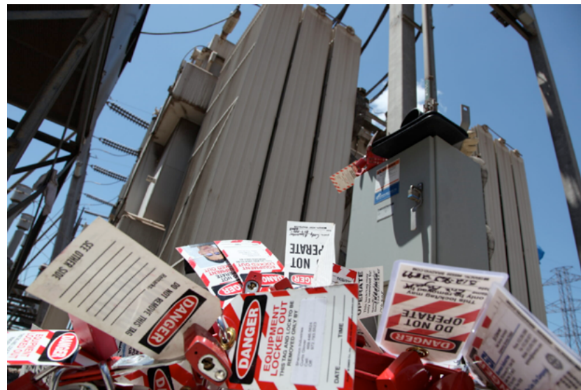
Figure 2: Locks and tags applied during a maintenance outage. Courtesy: Shermco Industries
