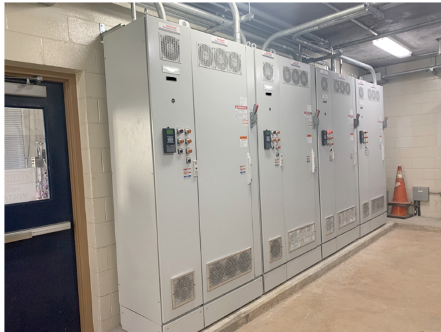
Figure 2: Variable frequency drives installed in environmentally controlled room. Courtesy: CDM Smith
